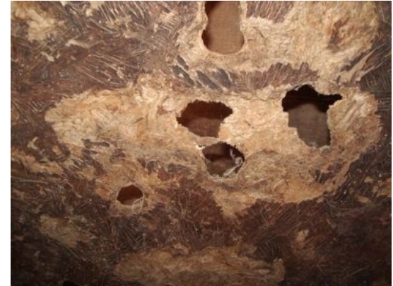
Particle board coop wall chewed by rats.
